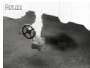
Gasleckagen an Armaturen
